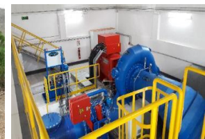
Turbine and Generator
