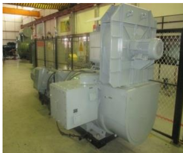
(MG Set for Testing Department)
