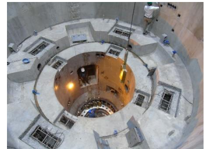
Figure 2: Broadlands Power House
